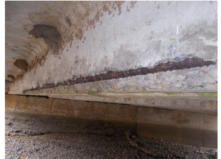
Eroding concrete girder
